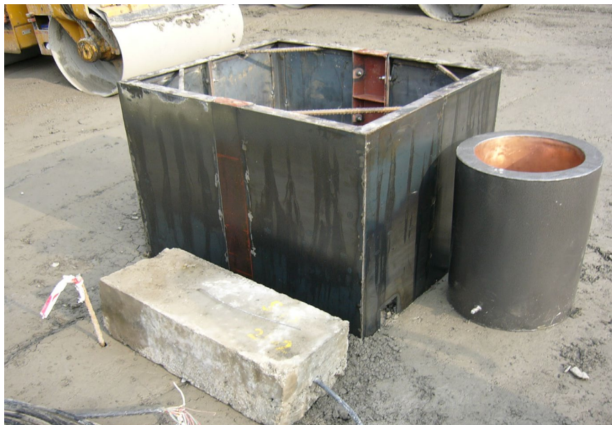
Fig 12: Formwork for installation of strain meter group at RCC dam site. The stress meter cast in a concrete block and the no-stress-strain container can also be seen.
