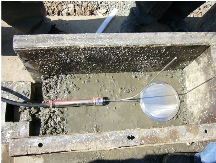
Fig11: Installation of stress meters in a concrete block to be later shifted to its location in RCC dam
