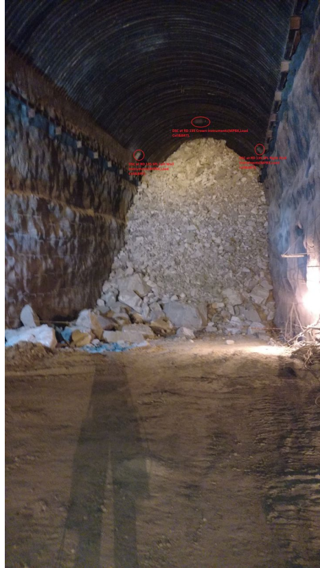
Fig. 19. Picture of the collapse (locations of the instruments are also indicated)
