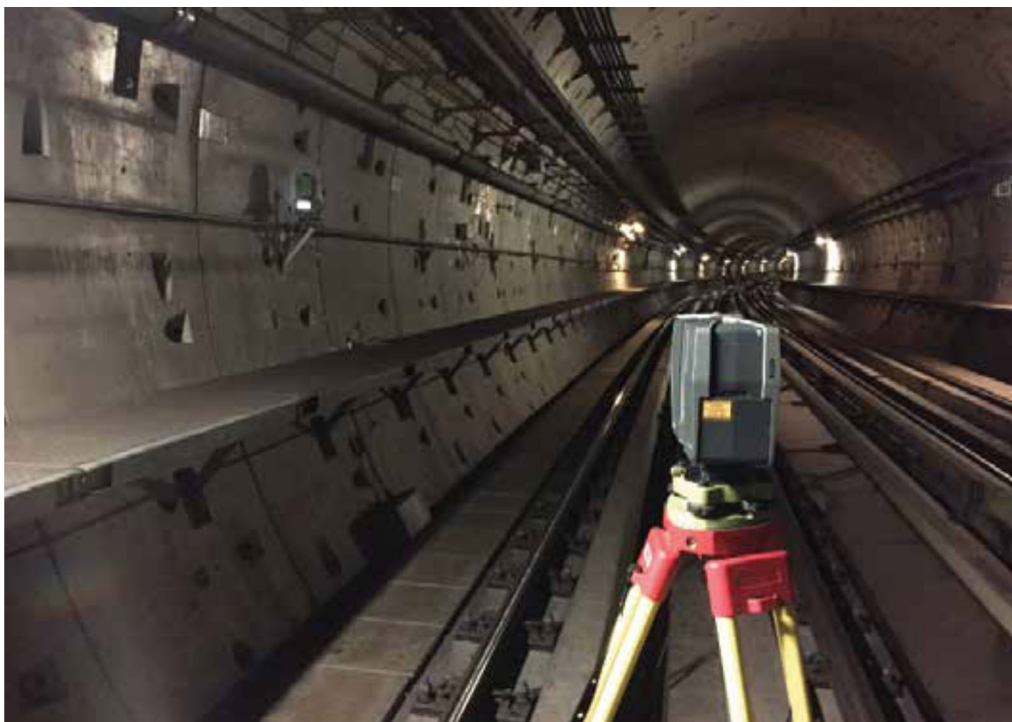
Fig. 12. Laser scanner for tunnel deformation monitoring
